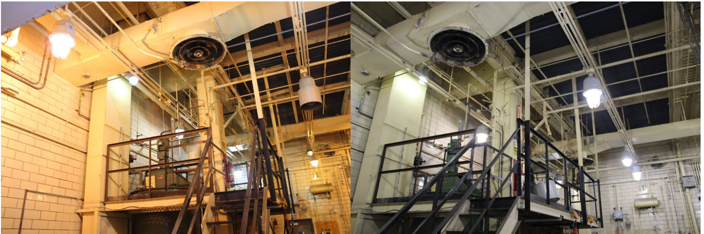
Before: 250W High Pressure Sodium Lamps
